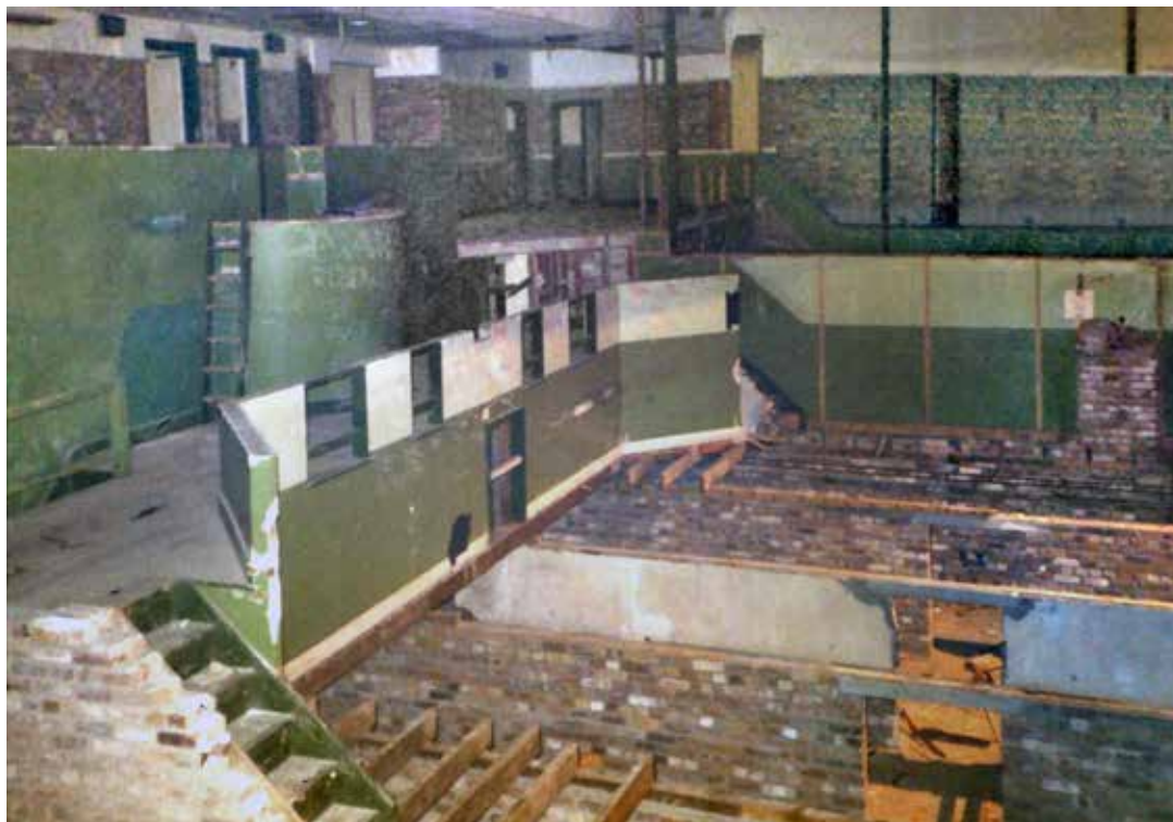
The operations room in January 1990 during the partial clearance of the building for reuse as a furniture warehouse. The picture was taken during a school trip by St. Andrews School. This image of the Ops Room clearly shows the Dais area and the foundations of the false floor; the image was taken from where the Filter Room was (see plan). The controller sat at the central curved fronted desk as indicated in the sketch. The naval plotting room was above the two-tone green wall to the right centre of image. Photo Kenny Ritch
